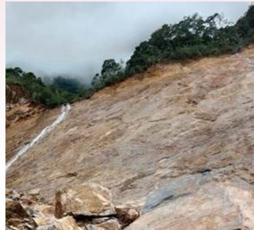
Figure 4: Planar failure in the crown area, note the presence of larger boulders and debris present in the crown is thread to buildings in the down stream area.
